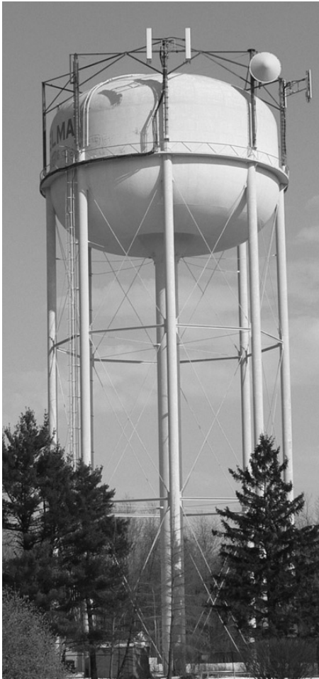
Elma Water Department will completely rehabilitate this 750,000 gallon water storage tank near Billington Road in the Town of Elma this summer. The project is being done to ensure good water quality within the system.
